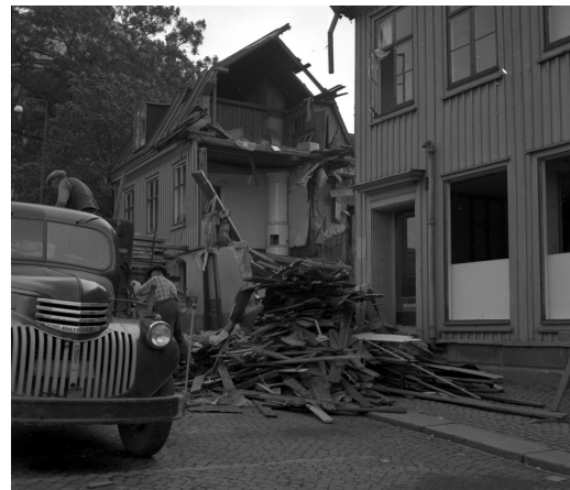
A wooden house from 1790 is being demolished to make way for the new City Library in 1957.
